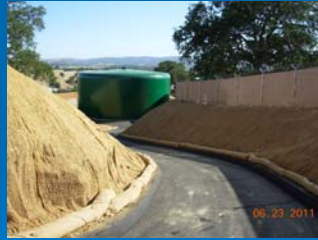
New 500,000 Gallon Water Storage Tank
