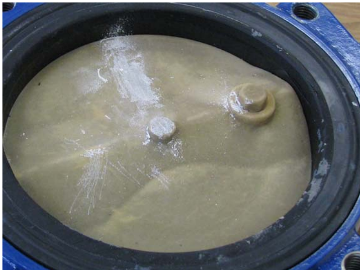
Photo 2: Excessively thick scale layer on the metal surface of a butterfly valve.
